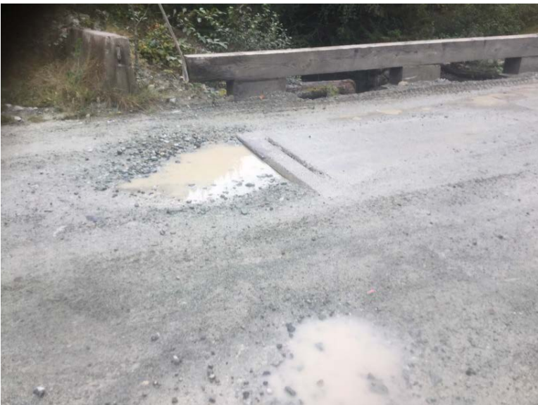
Pothole right approach
